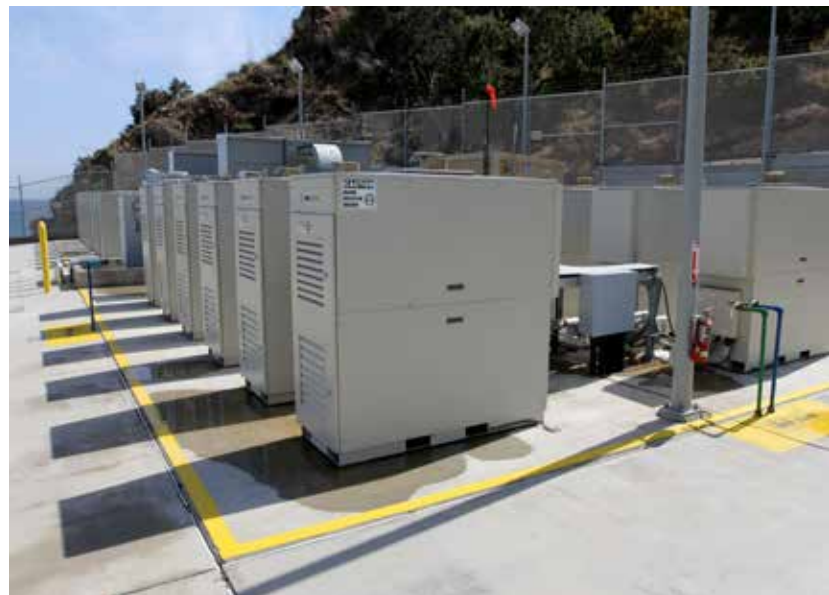
23 Capstone C65 microturbines provide prime power to Southern California Edison's Avalon site on Catalina Island.
